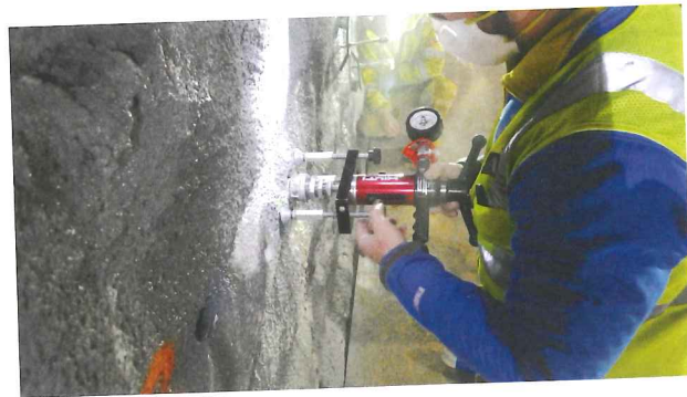
The 2-inch-thick overlay load tests Pull testing verified a good bond for the mix sprayed directly onto the existing blocks—a crew member applies pressure trying to pull away a cored circle of the overlay
