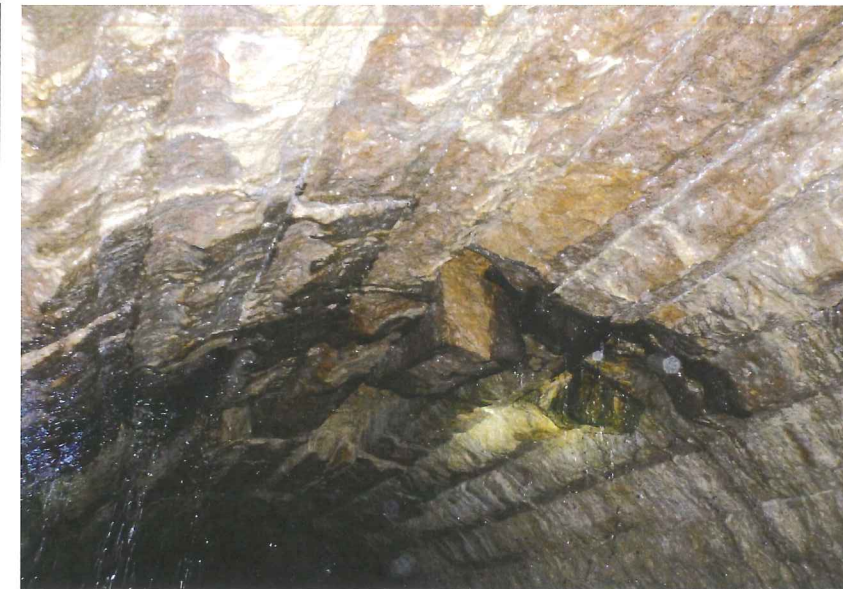
Above left: Damage to the limestone bricks
