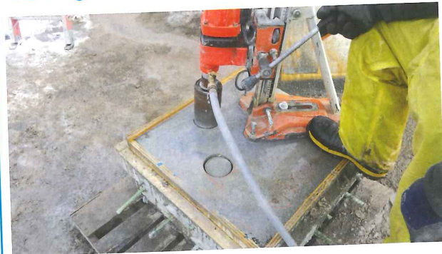
The 12-inch-thick overlay coring test panels Vertical and overhead test panels to certify the nozzlemen and their processes confirmed methodology and the absence of shadowing and voids
