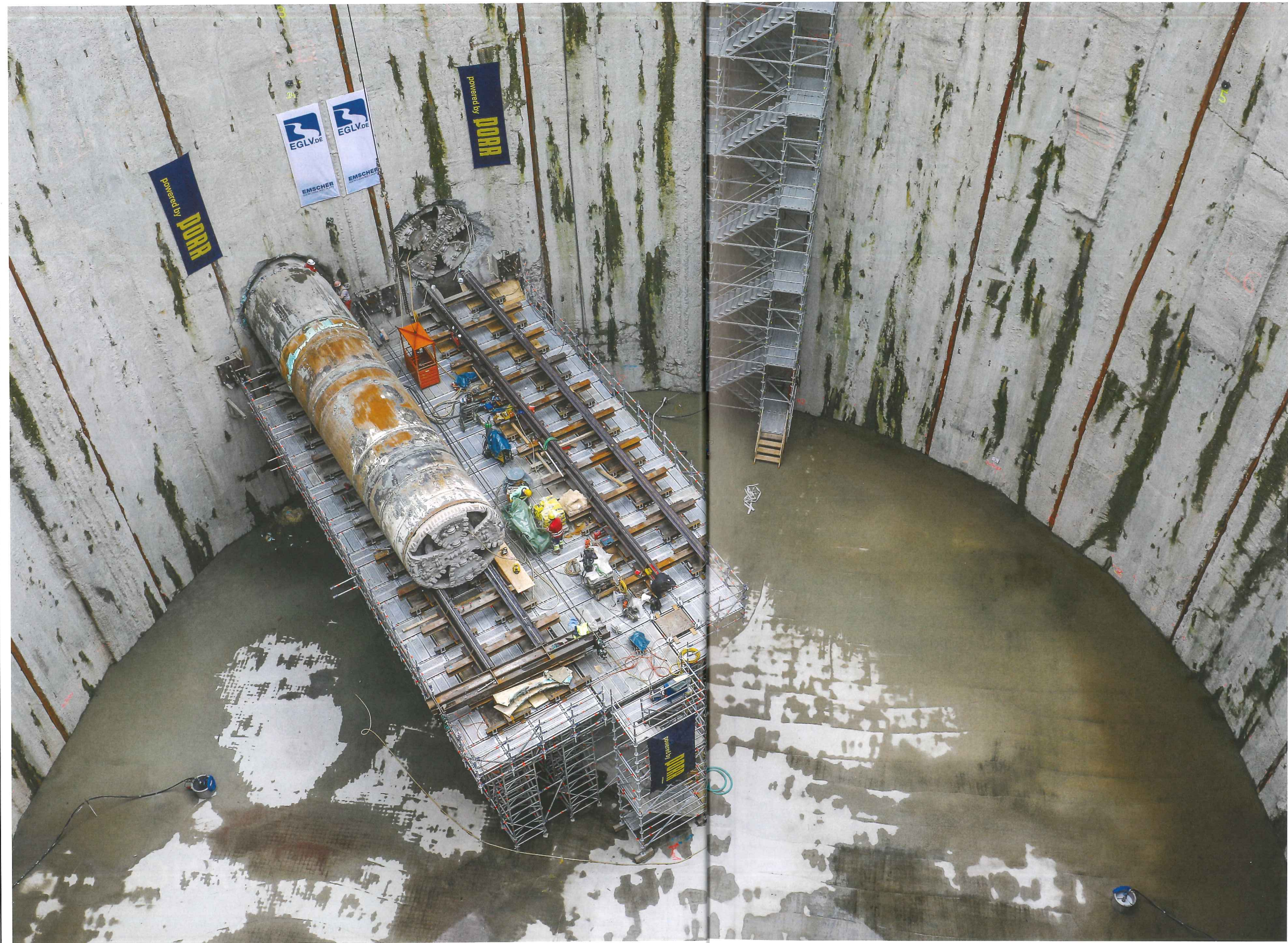
Left: With the support of Herrenknecht service personnel, between October 2014 and June two EPB shields (Ø 3,397mm) used by Porr on the Emscher Interceptor achieved performances of up to 177m per week and up to 582m per month. See news story, page 7
