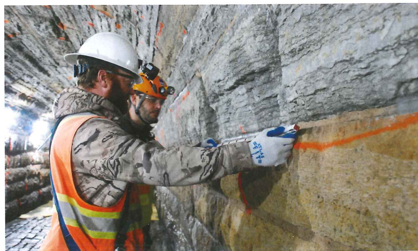
Below: Consultants measure damage in the tunnel
