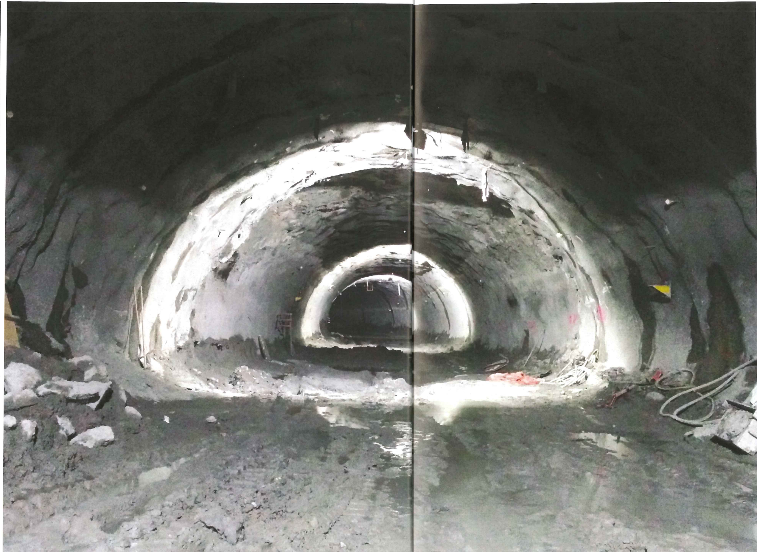
Left: Crews punched through on 28 December 2016, in Ottawa's LRT tunnel. The western portion of the tunnel has met the eastern portion, and there is now a contiguous 2.5km tunnel. Complete tunnel excavation is on track for the end of February
