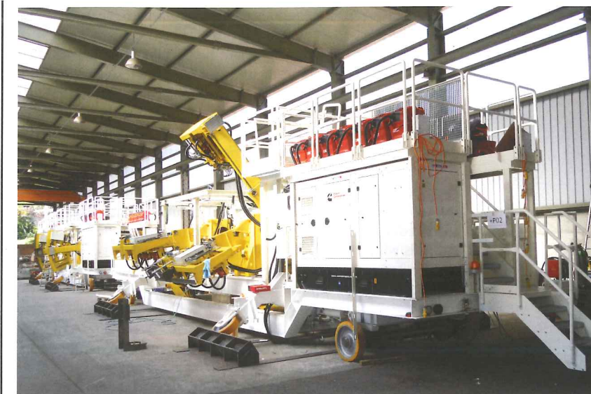
Above: Two Rowa rigs were used to drill the array of more than 250,000 holes required for services on the project
