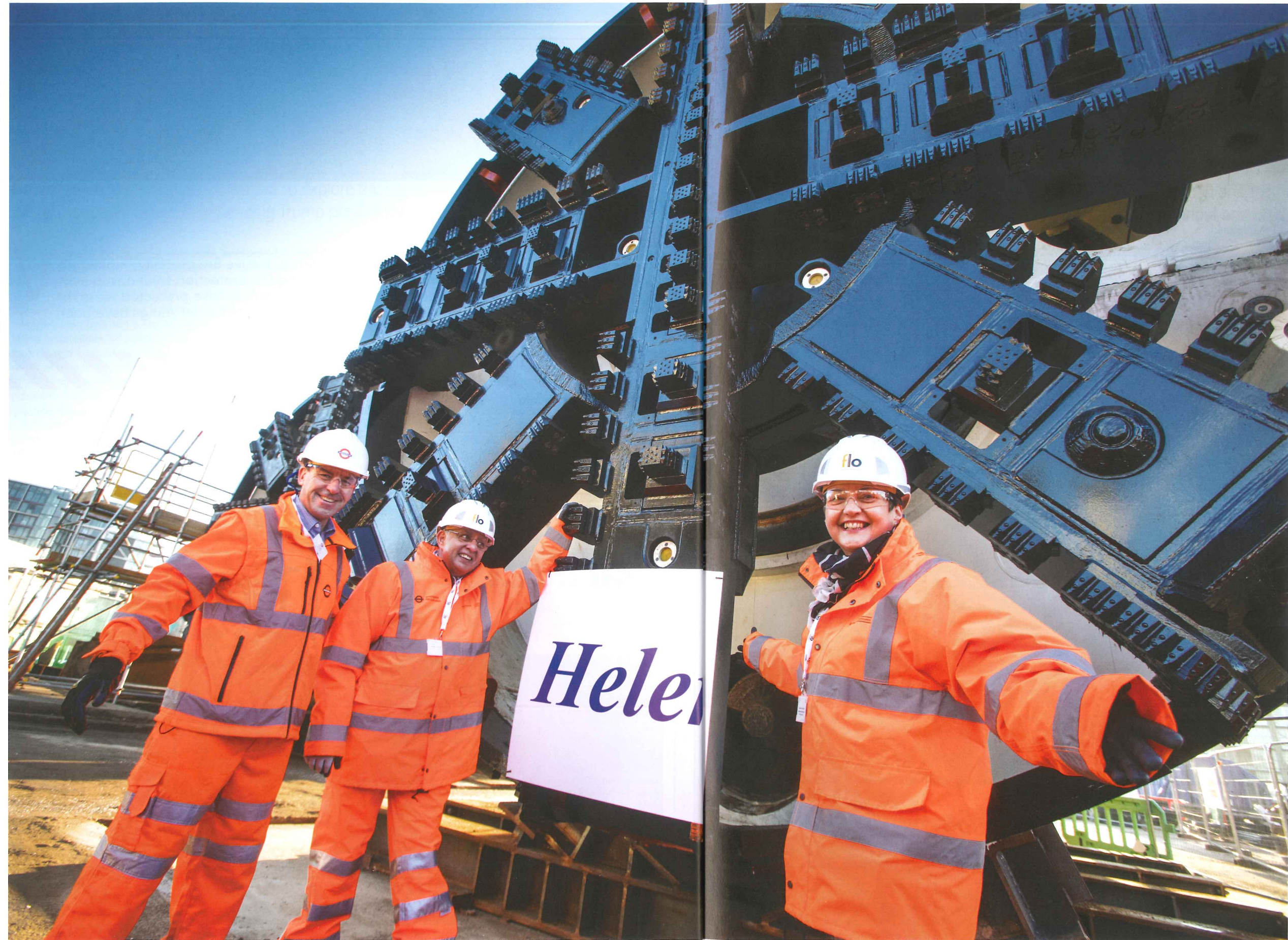
Left: A joint venture of Ferrovial Agroman and Laing O'Rourke (FLO) has revealed the two tunnel boring machines to be used in the Northern Line Extension project under South London in the UK. Read the full news story on page 8
