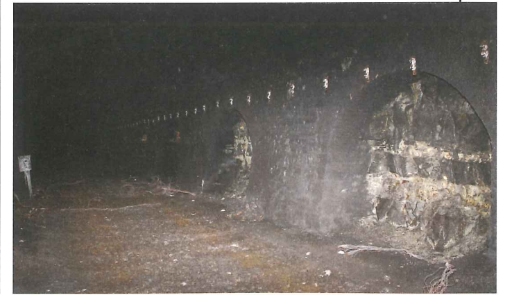
Below: The sidewalls and arches of this section of the tunnel are concrete
