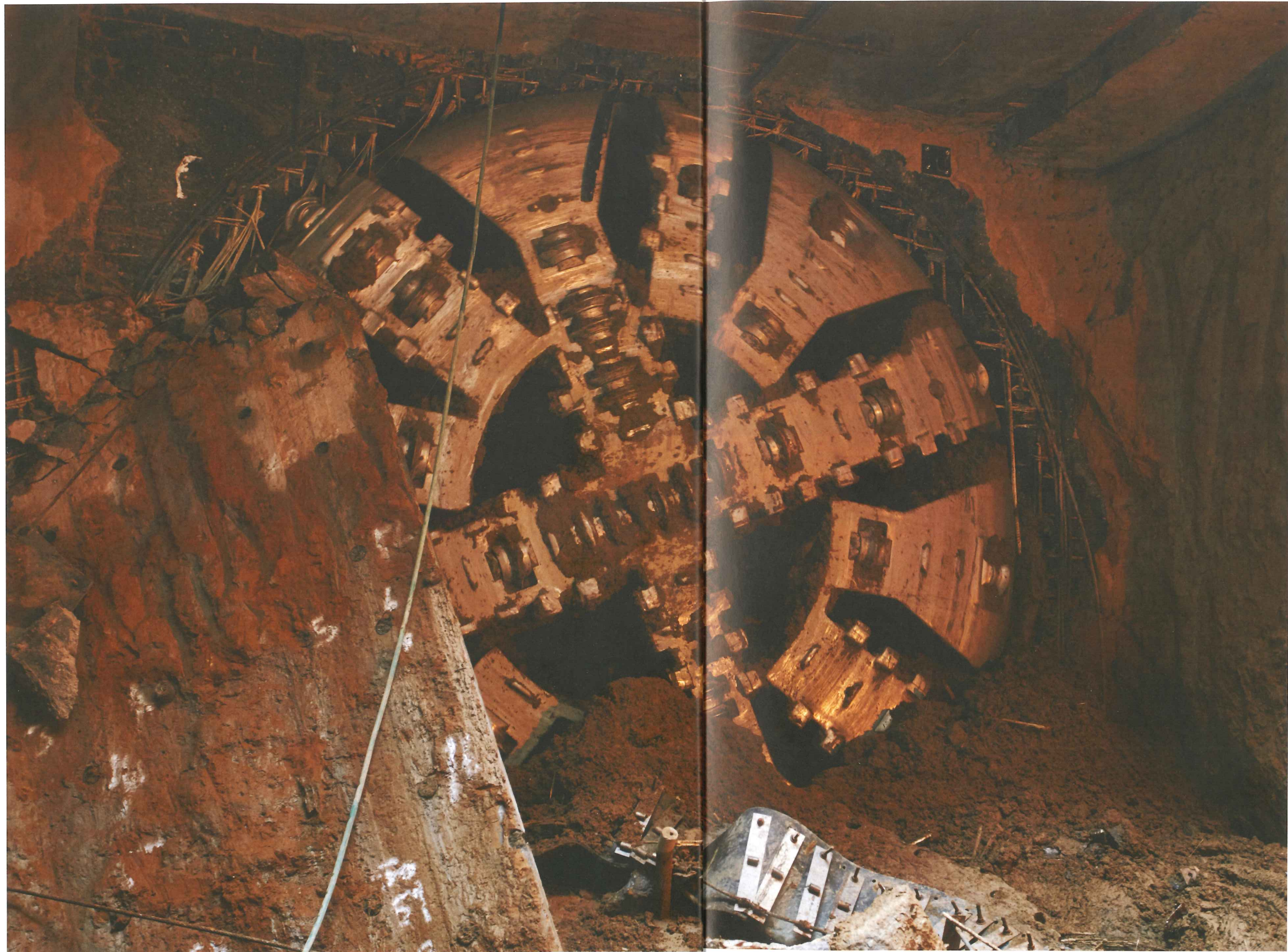
Left: Two Terratec 6.61m-diameter EPBMs made an historic double breakthrough on 14 November, marking the end of tunnelling works on the 58.6km Pink Line (Line 7) on Phase III of the Delhi Metro project in India
