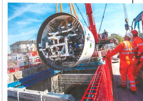
Right: The TBM launched this summer for the Shieldhall Tunnel in Scotland PHOTO: SNS PHOTOGRAPHY
