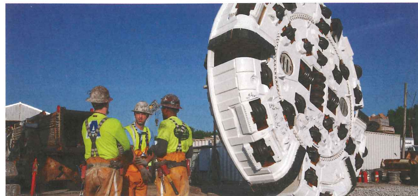
The TBM will have bored more than 51 km once finished with its Dig Indy tunnels
