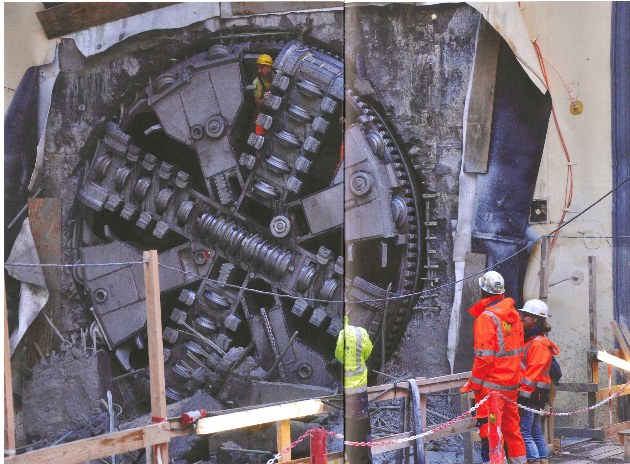
Left: Break through on the Copenhagen Cityringen Branch off to Nordhavn was achieved on 4 October. The TBM is captured at the moment of breakthrough on schedule into the reception shaft at Østersøgade following a drive of 1,900m from Nordhavn station. The machine contended with quarternary deposits under the railway then Copenhagen Limestone. Rambøll leads a joint venture with Arup as the client's engineer for this section
