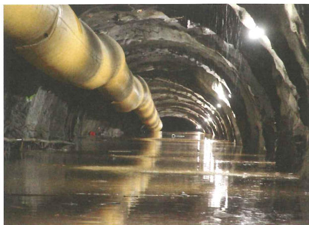
Above: Flooding at Vadlaheidi
