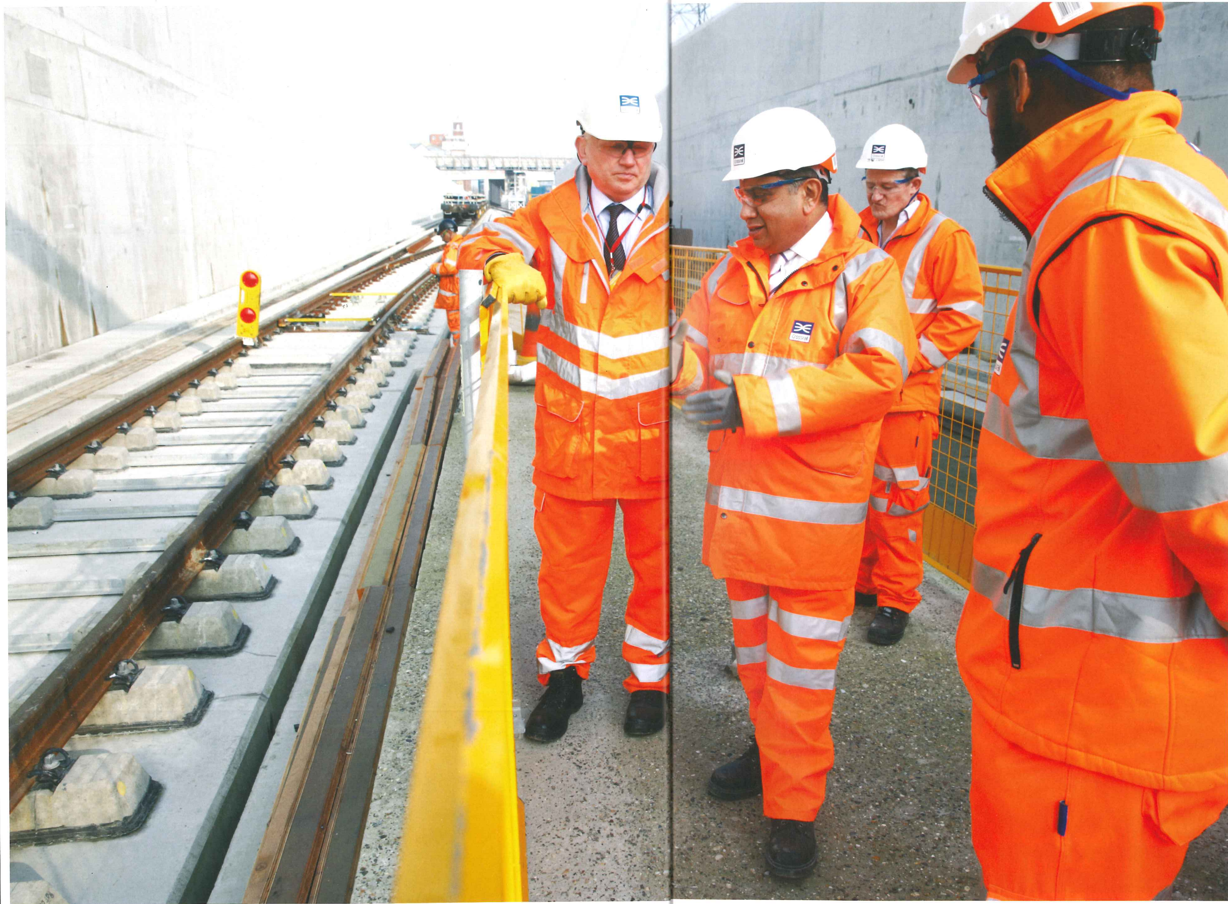
Left: Transport Minister Lord Ahmad has visited the Crossrail project to see the progress that has been made to install the permanent track in the new rail tunnels.
