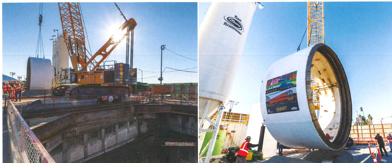
The TBM due to bore the Crenshaw/LAX light rail line was lowered in early March
