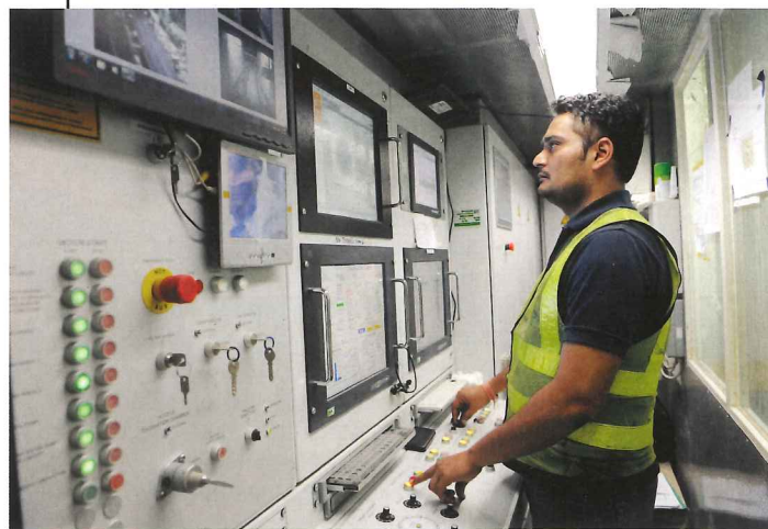
Below: TBM control cabin with operator
