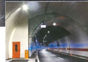
March 1st Tunnel Bosnia and Herzegovina First 100% LED tunnel lighting solution in this country
