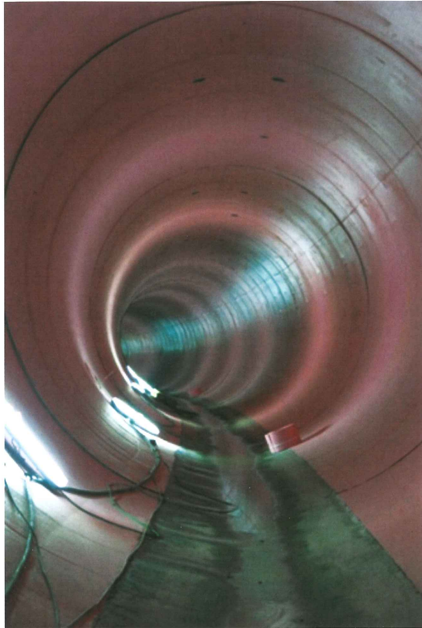
Above: Corrosion protection lining on the main tunnel
