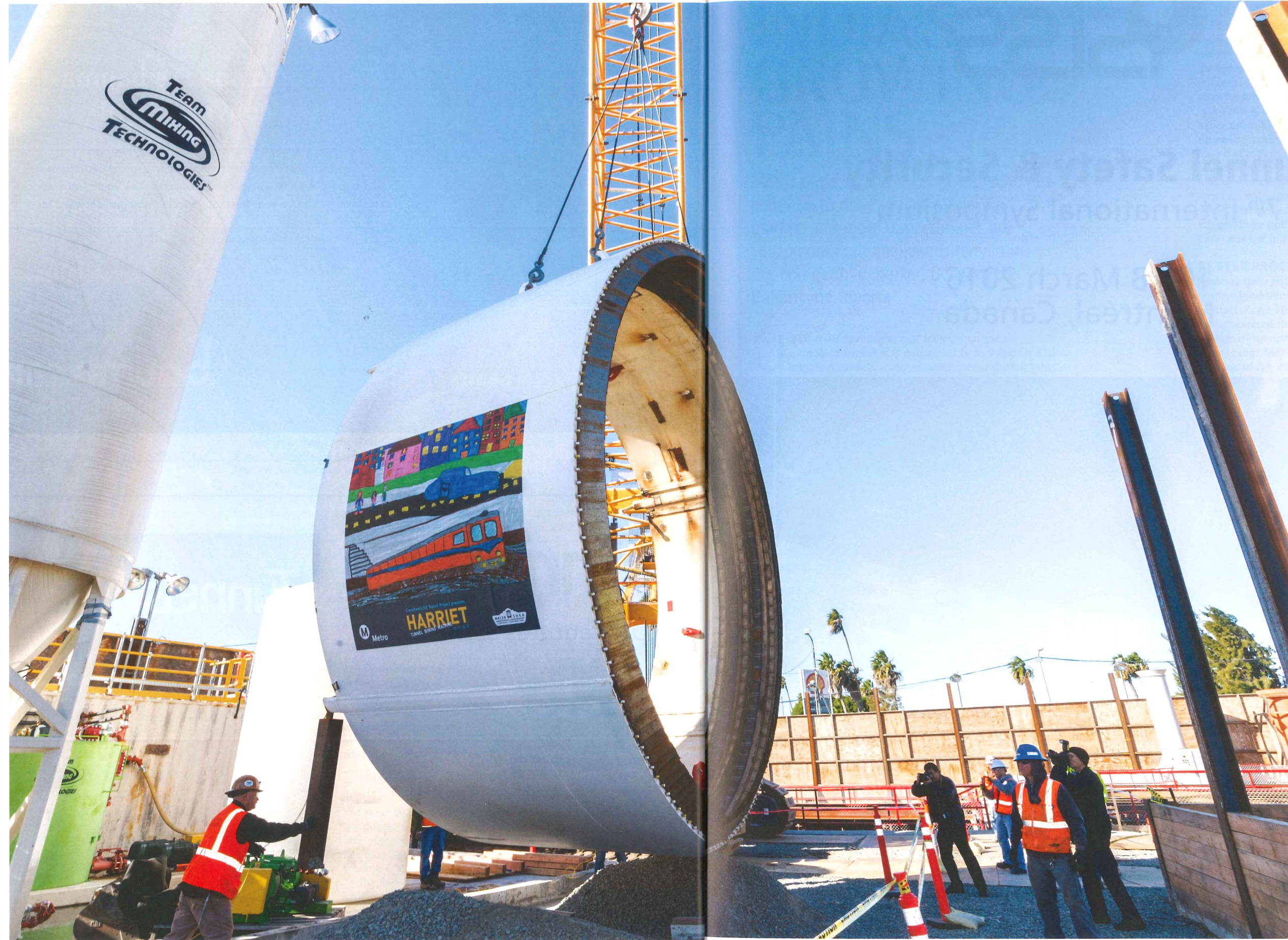
Left: The Los Angeles County Metropolitan Transportation Authority (Metro) held a TBM lowering ceremony on February 1 for the Crenshaw/LAX Line. The TBM, a 6.5m-diameter Herrenknecht machine, will excavate twin 1.6km tunnels at the northern end of the new rail line. The 13.7km Crenshaw/LAX Line is a USD 2.058bn light rail line that is being built by Walsh-Shea Corridor Constructors, comprised of Walsh, Shea, HNTB, Comstock and Arup. It is expected to open in 2019
