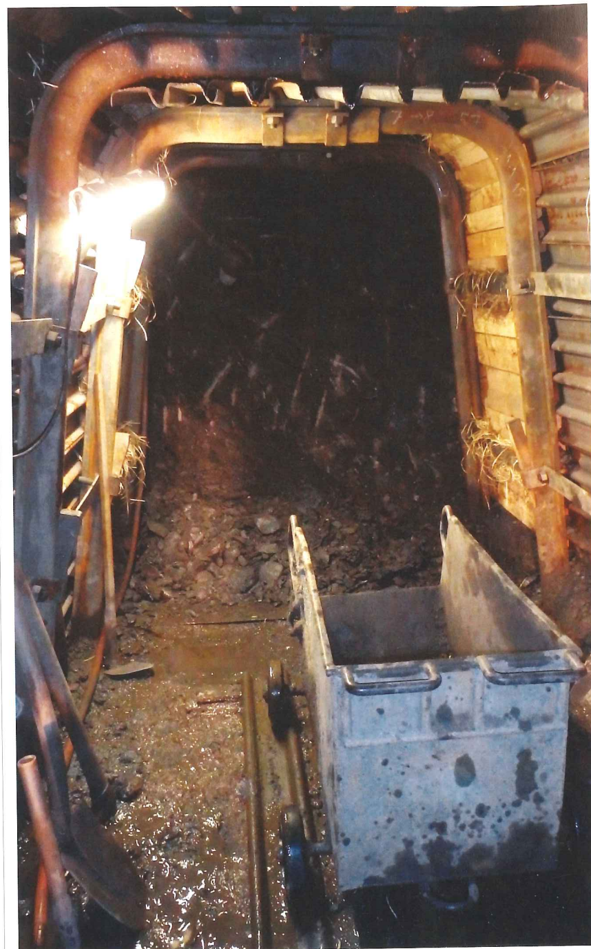
Above: Initial lining of the trapezoidal steel mine support frames in stable ground - lagged/ timbered tunnel walls (Interceptor Sewer 'H' in Prague)
