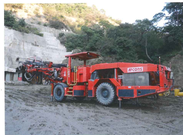
Afcons built four twin tube road tunnels each 1.5km long over a 65km length of highway with DT820s
