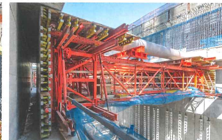
The VARIOKIT traveler system rolls from one section to the next on rails after each pour, without the formwork having to be broken down and reassembled.
