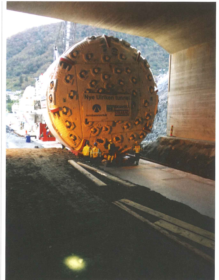
Above: The TBM approaches the face on the Ulriken Tunnel, article on p.46
