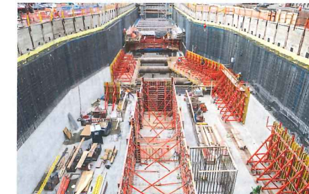
The formwork solution is based on system components of the VARIOKIT engineering construction kit. The traveler system for the bottom level is also used in the upper levels.
