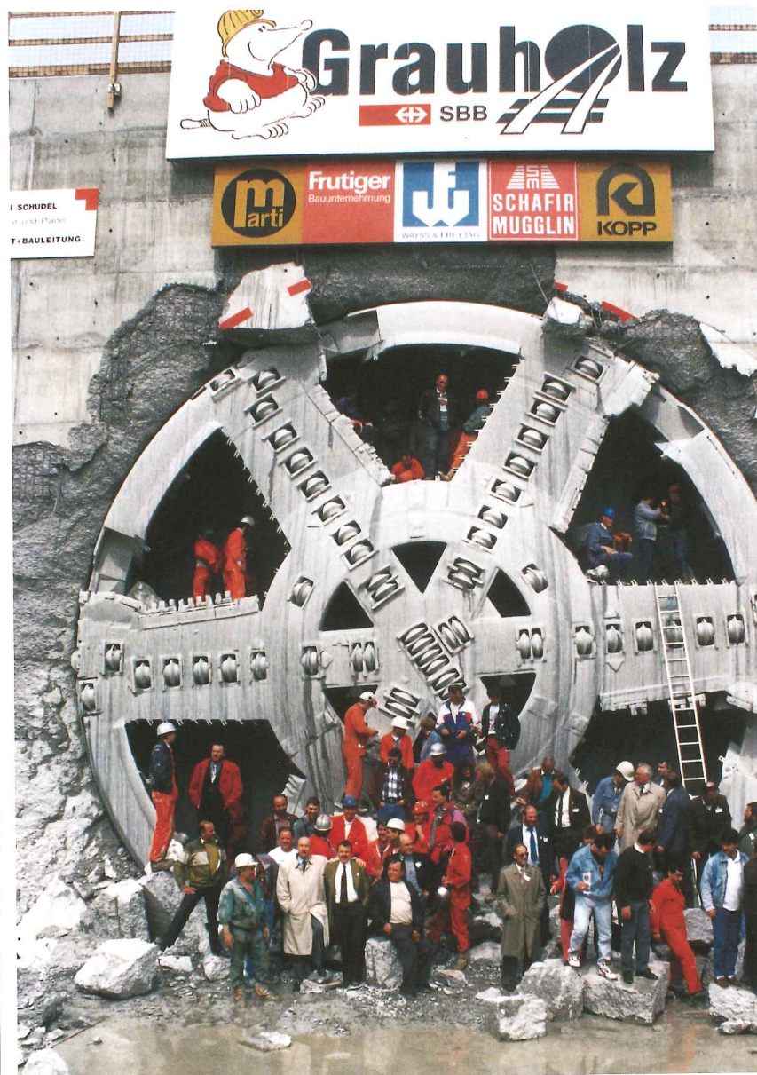
Above: In 1988, the Mixshield surpasses the 10m mark with this 11.6m machine destined to excavate the Grauholz Tunnel in Switzerland
