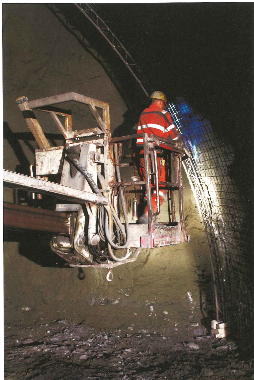
Below: Progress has been painstaking in places, but water ingress has been less than expected
