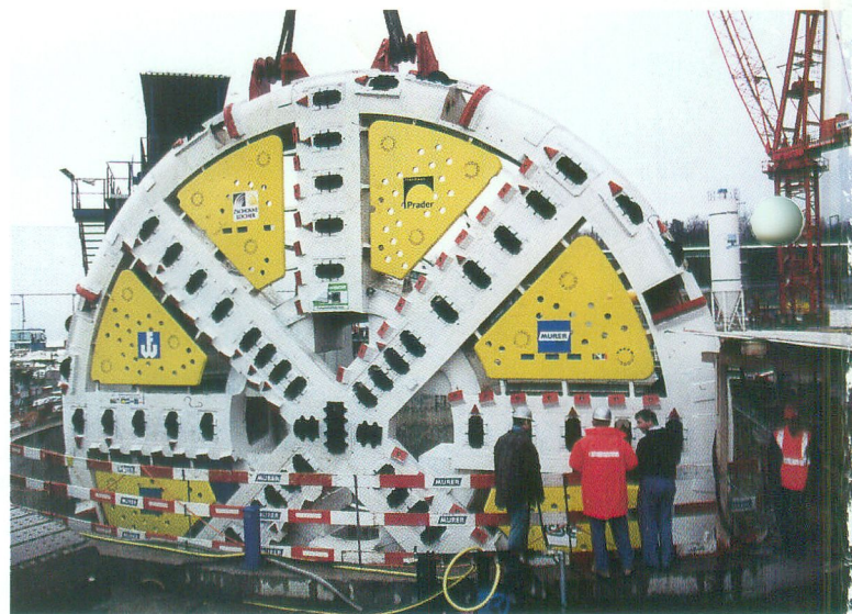
Two newly constructed Herrenknecht machines are being implemented in the Zurich-Thalwil project: The record setting TBM (12.29m diameter) and a 12.39m Mixshield (photo). Tunnelling with this from TBM to slurry convertible machine has commenced on March 31 st .
