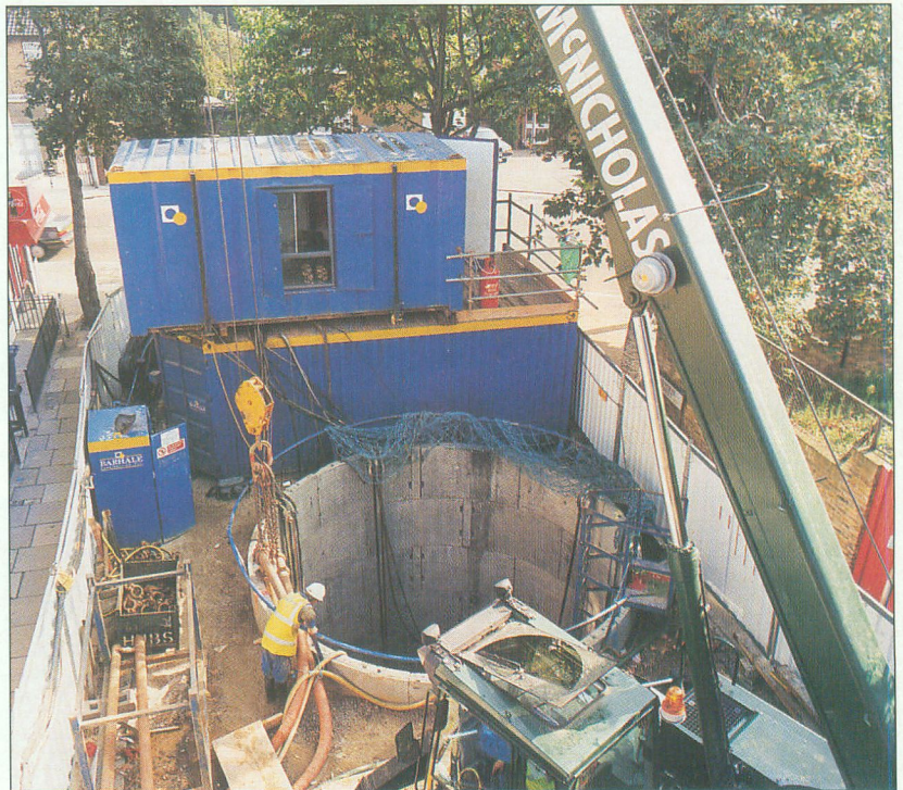
Joint venture plant in use at the Unclemole drive shaft (21) in Admiral Street
