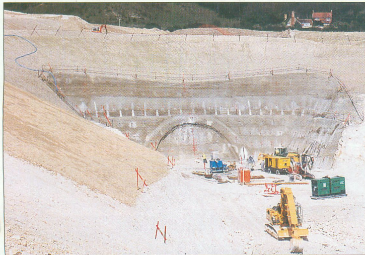
The Country Portal Site of the North Downs Tunnel, part of package 410 of the Channel Tunnel Rail Link
