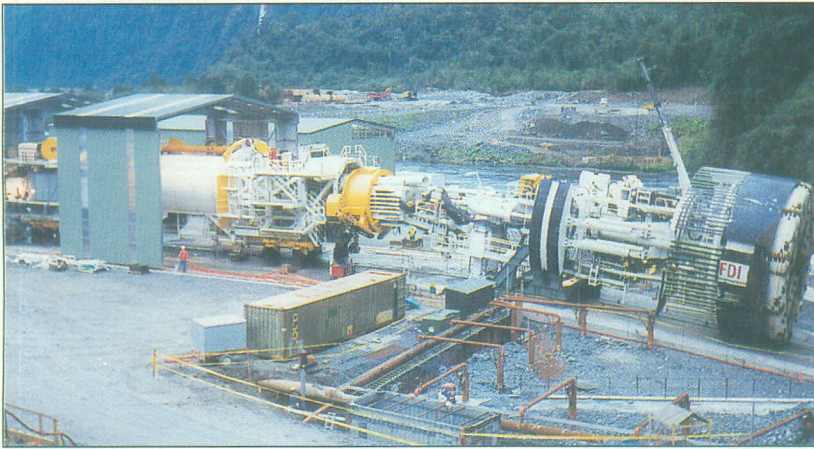
The Robbins TBM323-288 and Rowa back-up 'walking' down the 12.5% decline to the tunnel face
