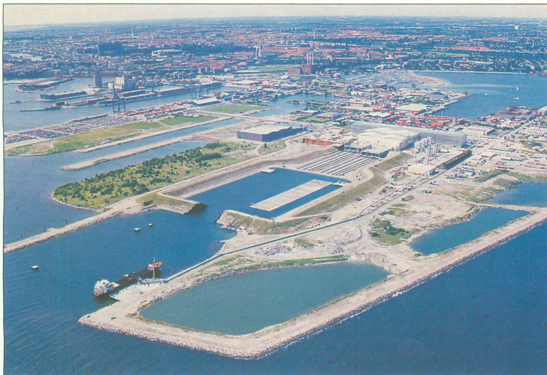
Overall view of the casting complex for the Øresund immersed tube tunnel
