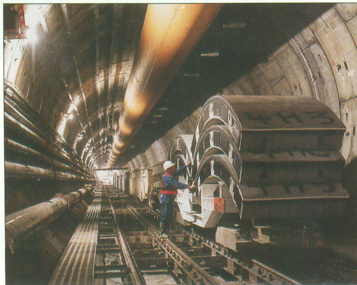
Work under way on one of the marine running tunnels for the Channel Tunnel
