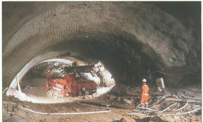
Jet grouting for the umbrella arch in the Ristet off ramp tunnel to allow excavation in soft ground
