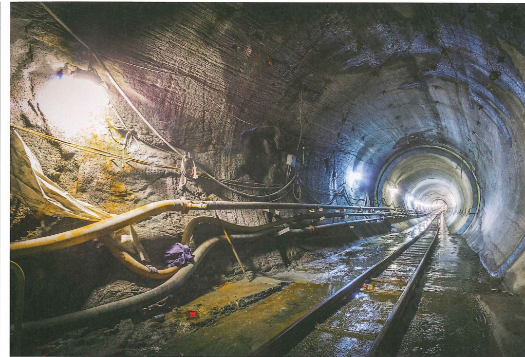
Left: All excavation on New York's East Side Access project has completed PHOTO: MTA
