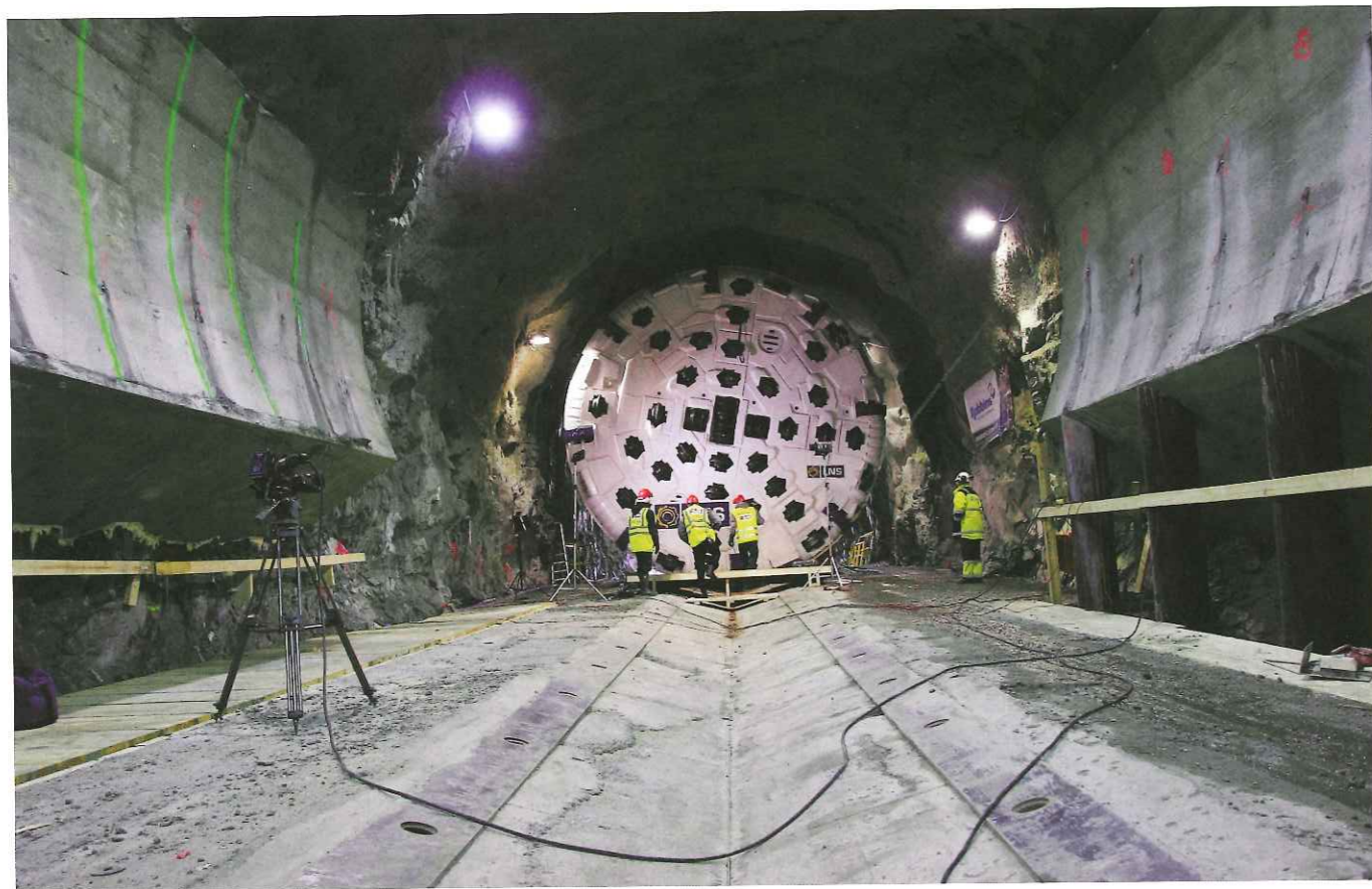
Above: Norway's first TBM in 22 years, a Robbins Main Beam, was launched on 16 January 2014
