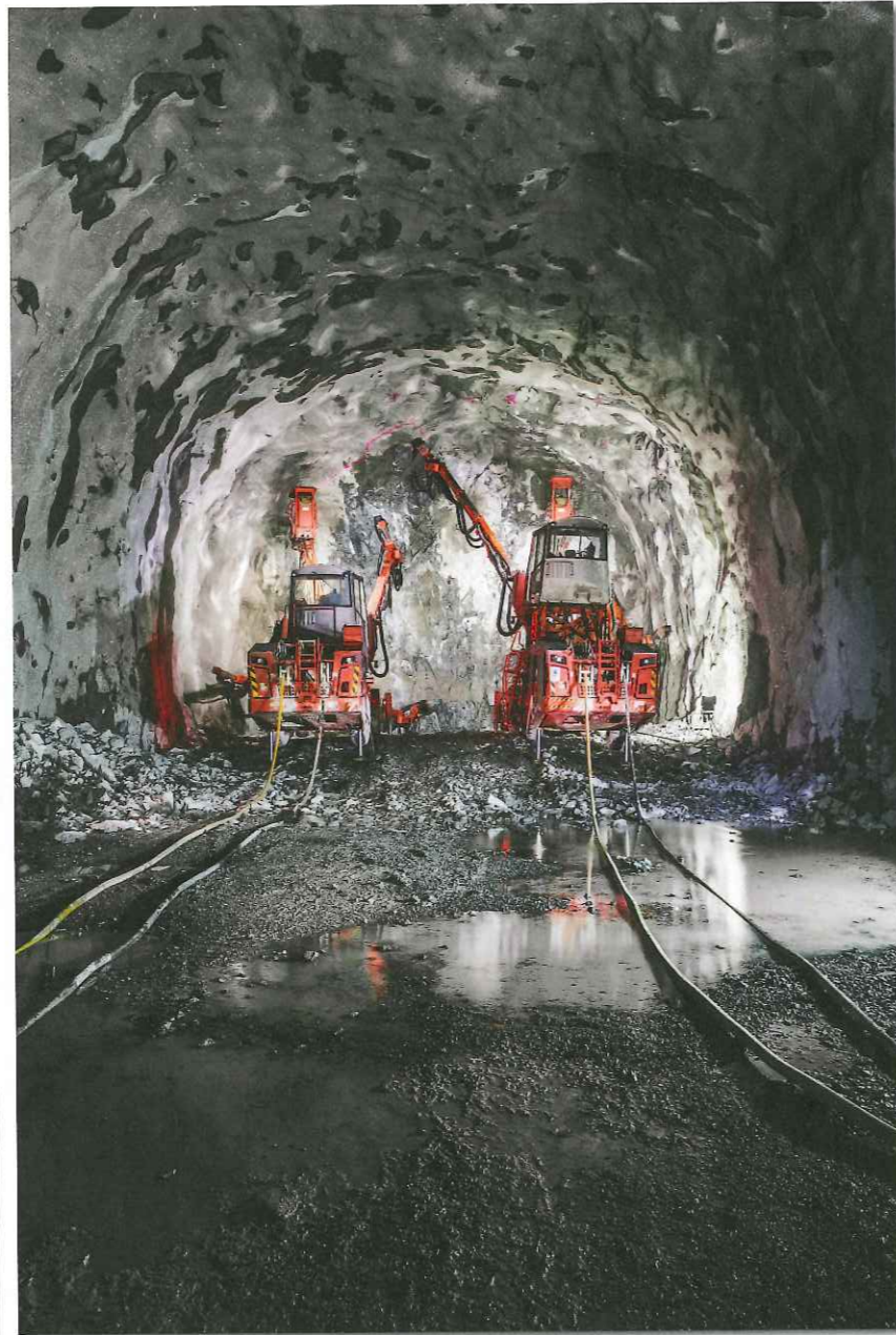
Above: Drill rigs working in concert, allowing for faster advance over a greater excavation area
