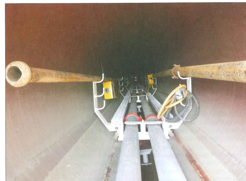
Above, top and bottom: View into and cross-section of a 48in pipeline with supply lines placed on movable support structures
