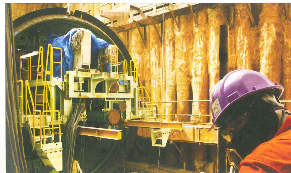
Above: Bangalore's first TBM, Helen, was due to break through shortly after Tunnels went to press
