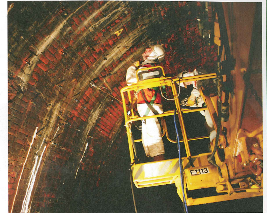
Above: Inspecting for any remaining seepage following installation of polyurethane resin through the packers shown
