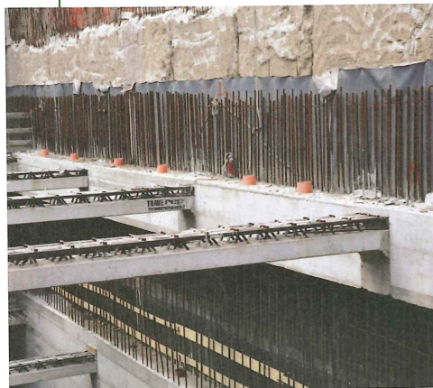
Above: Soprema sheet waterproofing membrane used in cut-and-cover tunnelling for Line C of the Rome Metro
