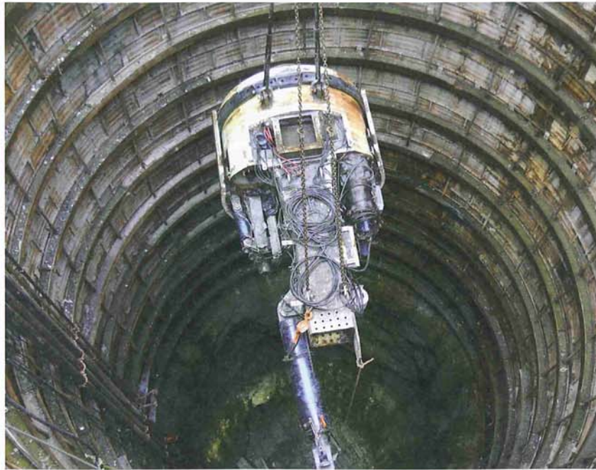
Above: The Renda/Southland JV broke through into an intermediate shaft in November 2010, and then removed some TBM components for launch in the opposite direction.
