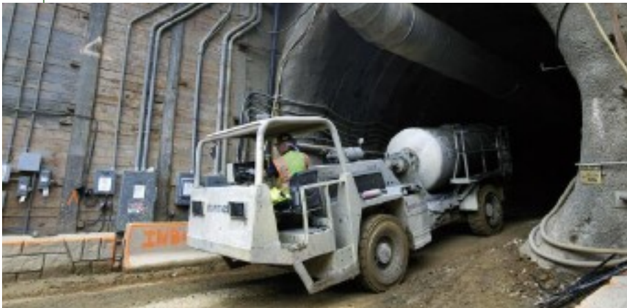
Left: A Normet Utimec low profile truck mixer emerging from a tunnel on Washington's Dulles Metrorail Corridor project
