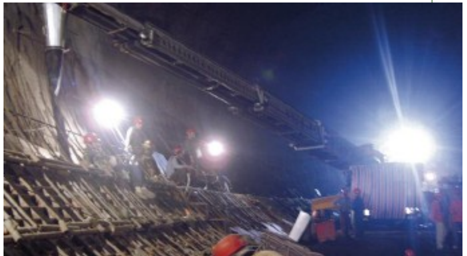
Above: A Putzmeister Telebelt is used for concrete placing on tunnels of the Xiluodu hydroelectric project on the Yangtze River in China
