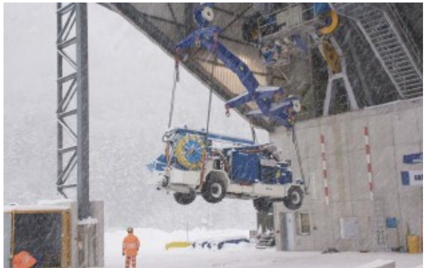
Above: A Meyco Potenza concrete spraying system was transported by a Garaventa cableway to excavations for the Linthal 2015 hydroelectric project refurbishment scheme
