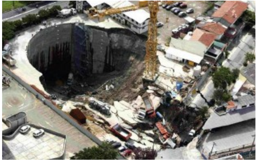
Above: The Pinheiros station cavern and shaft collapse in Sao Paulo in January 2007
