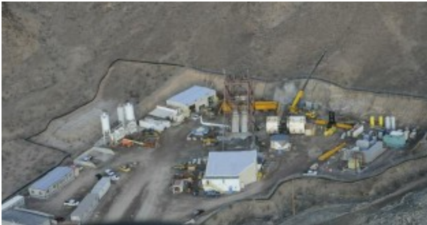
Left, top: Another Liebherr Easymix 1.0 is used at the Lake Mead No. 3 tap tunnel project by Vegas Tunnel Constructors. Here it occupies a small footprint (left centre) within the working shaft site;
