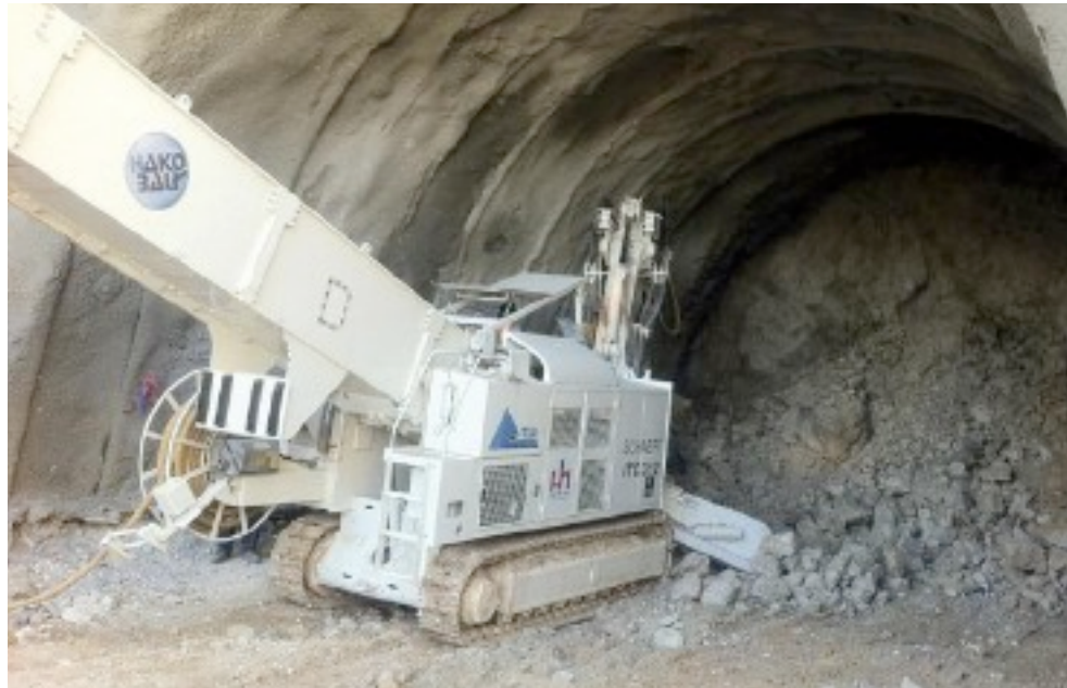
Above: Spoil removal with a Schaeff ITC 312 loader at first tube of Tunnel 3A
