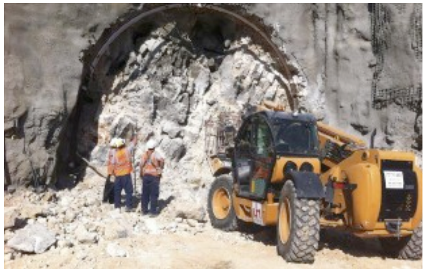
Above, top: Map of the fast rail link under construction in Israel Above, bottom: Initial groundbreaking at second tube on Tunnel 3A
