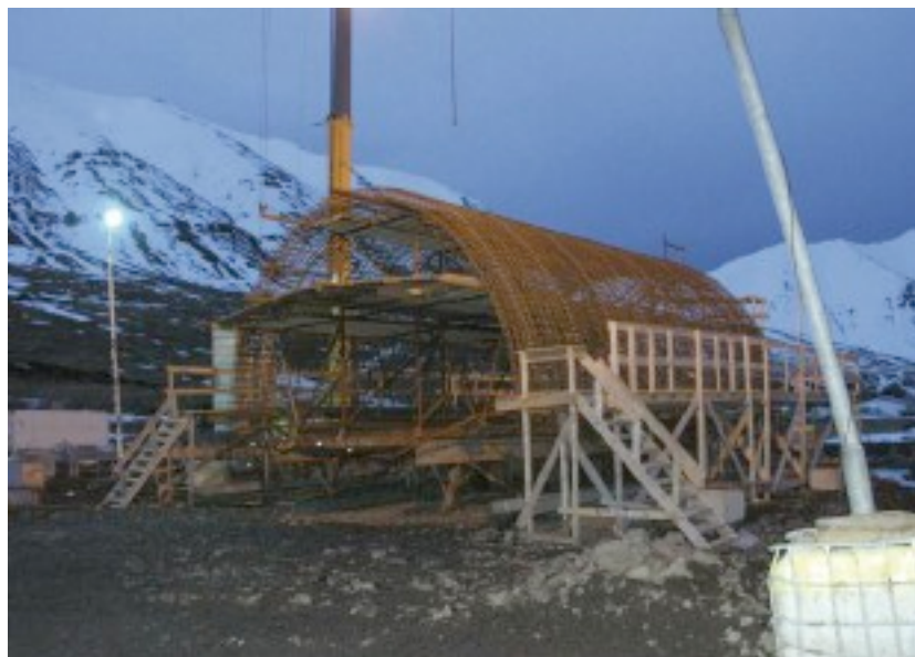
Above: Olafsfjordur Tunnel, at the south east end at Olafsfjordur town, where steel reinforcement was being assembled at the end of 2009 using a multi-platform gantry arrangement on a flat wagon to help with insitu concrete portal construction
