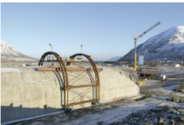
Above: Portal construction at Olafsfjordur in its final stages in February 2010, with the outer formwork removed while the inner formwork remains in place.
