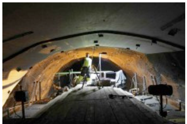
Above: A new survey, calculation and organisational system was developed to speedily undertake installation of each individually-sized WFP positioning bolt at Hedinsfjordur
