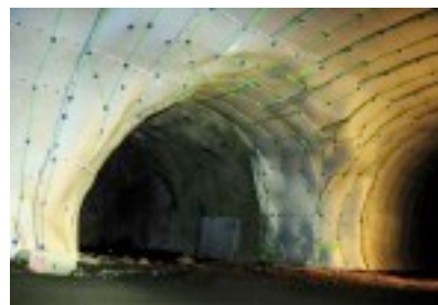
Left: Difficult geology and groundwater ingress were significant aspects of drill and blast construction of Hedinsfjordur scheme, particularly on parts of Olafsfjordur Tunnel, which at 7,150m long (including portals) is also the longest, single tube, uninterrupted road tunnel in Iceland
