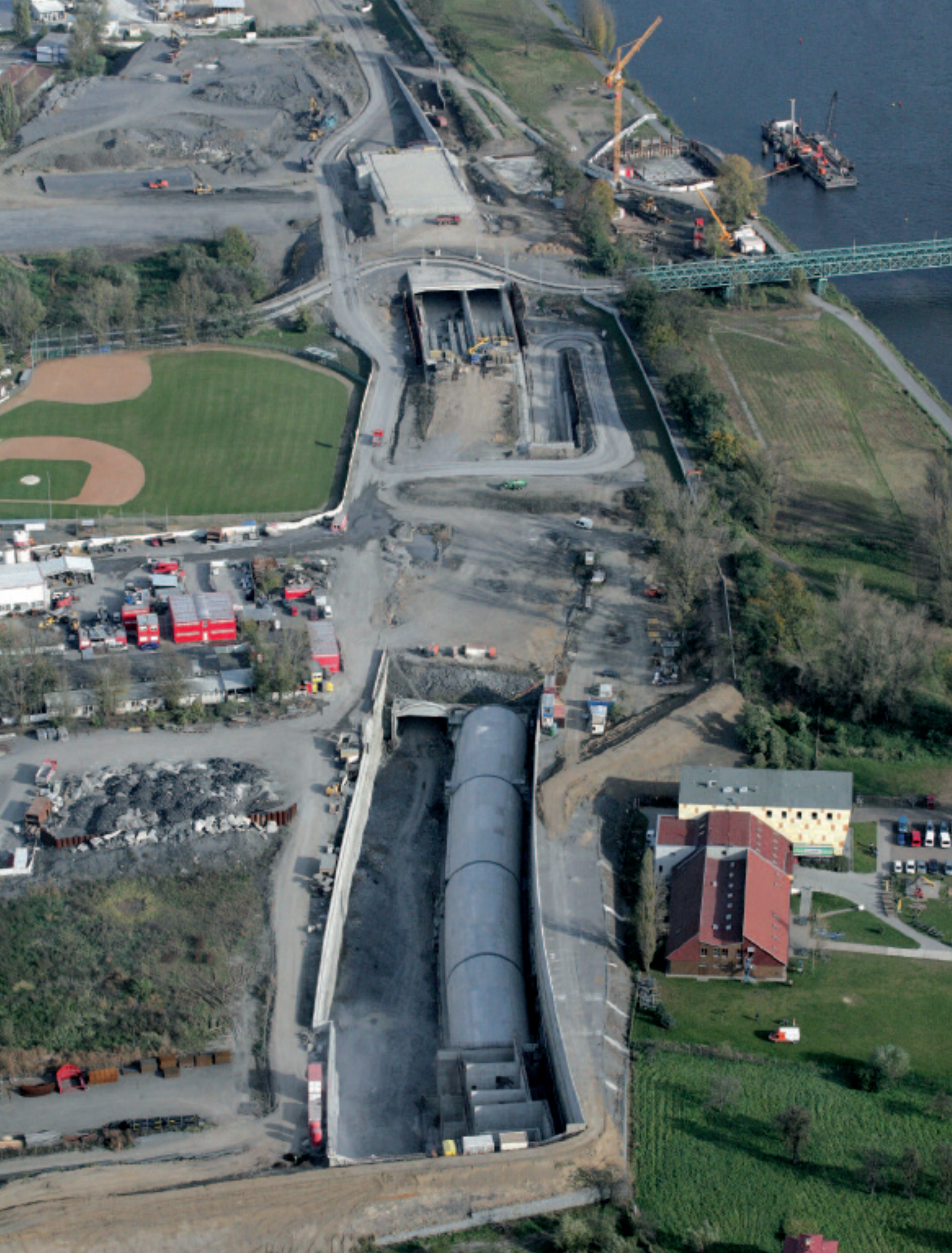
The Blanka complex of tunnels in Prague is the largest underground construction project currently underway in the Czech Republic.
