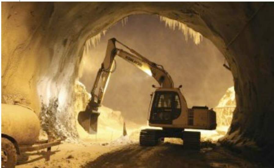
Right: Outside the water froze and it snowed, inside the tunnel and the work went on
