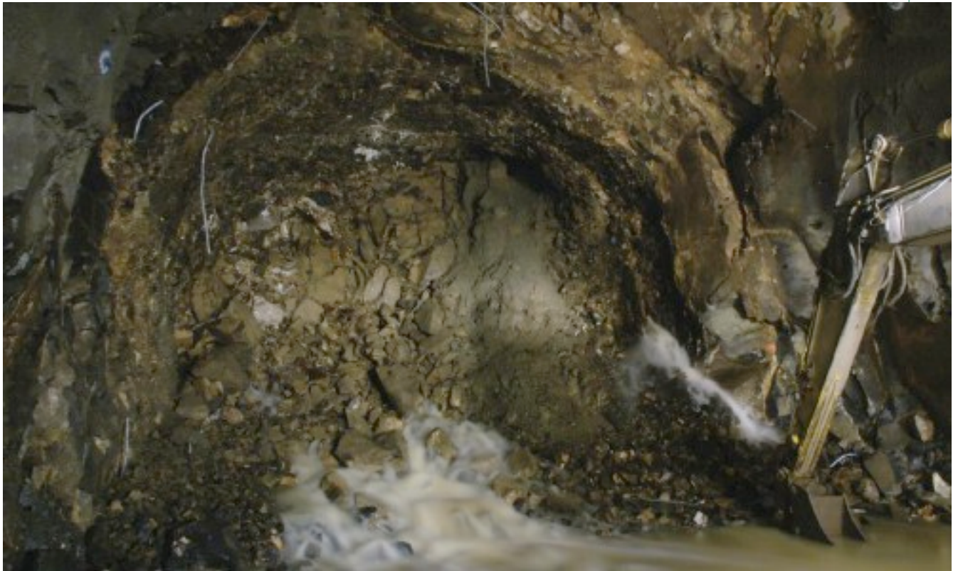
Above: The severe groundwater problems sometimes seeped and soaked the excavation face ...
