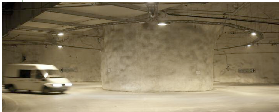
Above, left: Image 5: Hi-Fog spray head system installed in roundabouts in Helsinki service tunnel;
