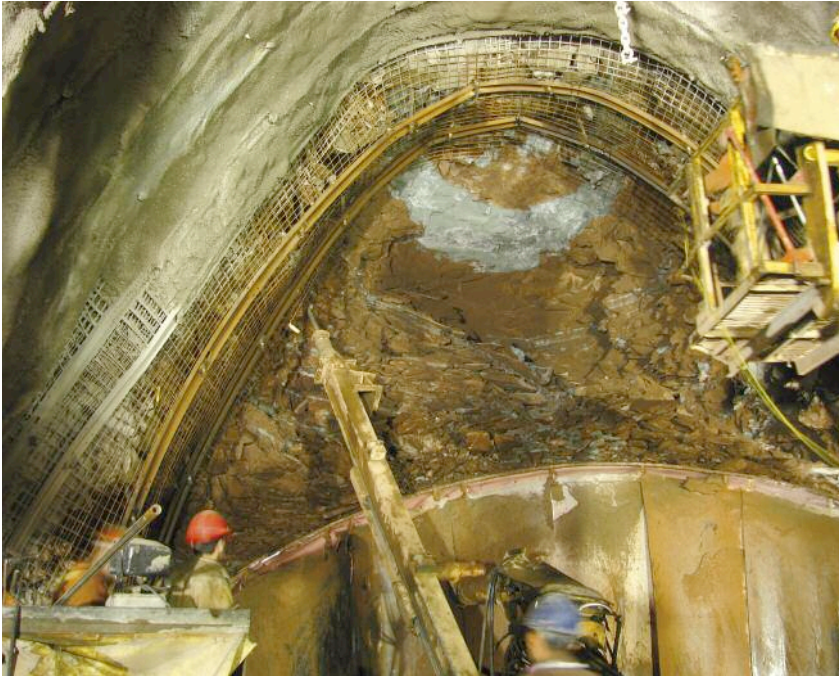
Left: Extreme overbreak while boring has led to a new route for the tunnel
