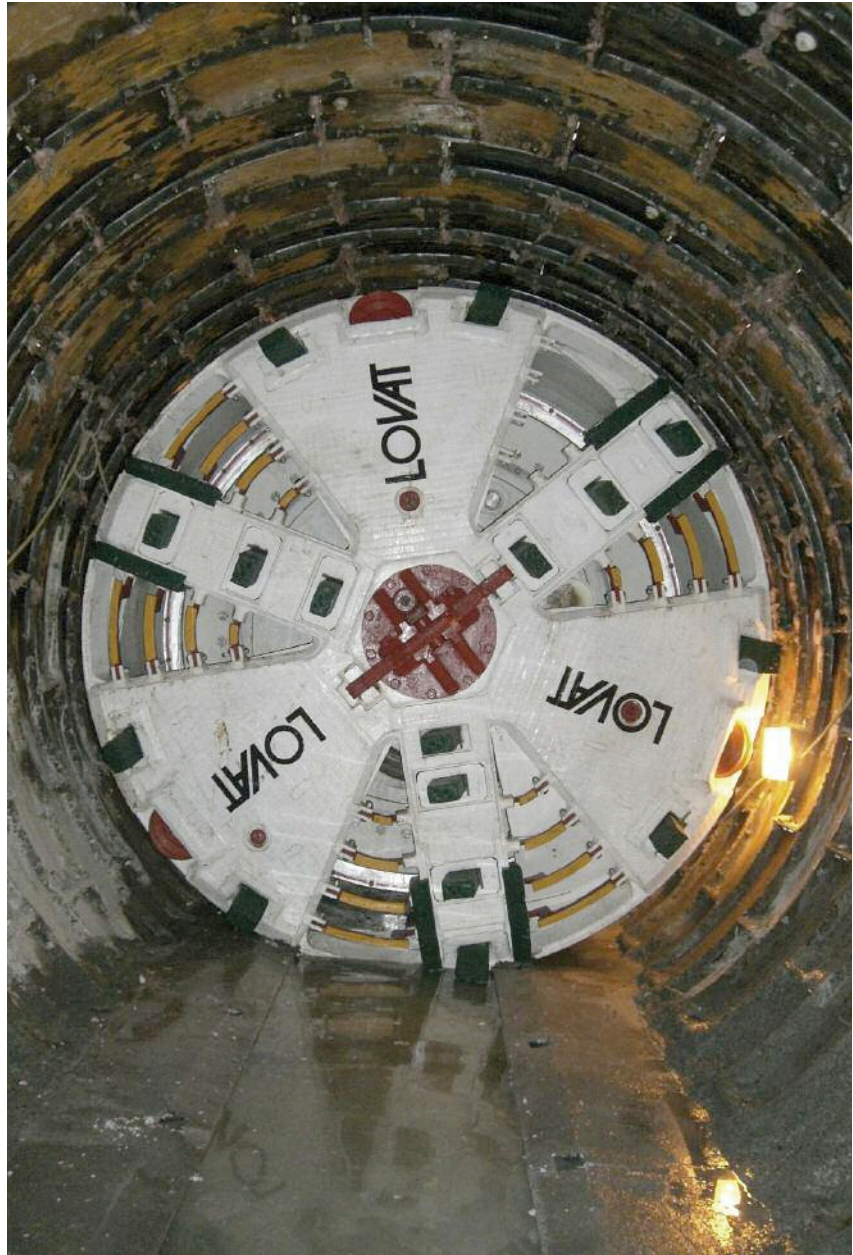
Above: The 2.6m diameter EPBM will cut through glacial tills and waterlogged sand
