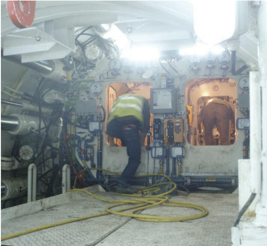
Left: The front of the TBM is a squeeze with two man locks needed to speed maintenance works
