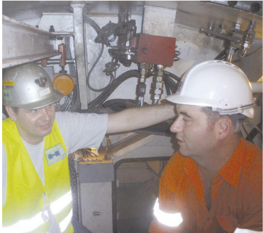
Above: Herrenknecht country manager Thorsten Gartner speaks with Leighton Contractors project manager Piers Verman in the pressurised chamber at the front of the TBM before launch
