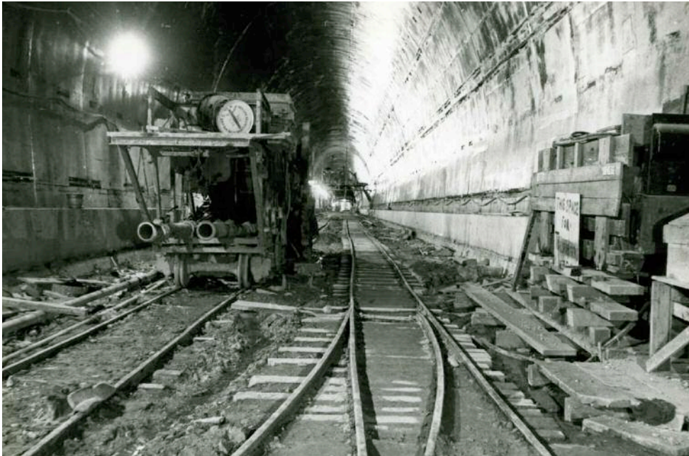
Left: A view of construction on the first bore of the Caldecott
