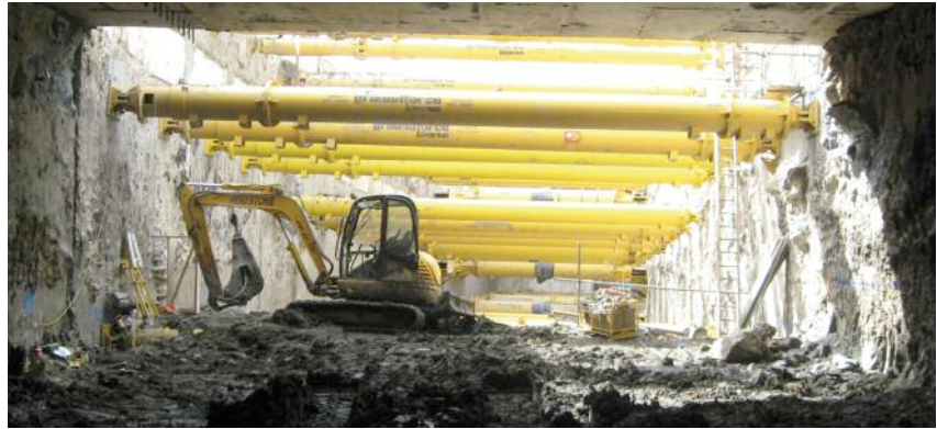
Above: Several excavation methods were used, including cut-and-cover with temporary support struts removed as construction proceeded
