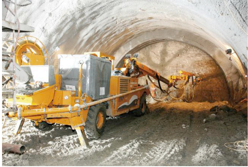
Above: One of two Putzmeister-Sika SPM 500 PC wet-spray concrete manipulators used on the B29-Schwäbisch Gmünd bypass tunnel for a thick shotcrete lining sealing below the water-table.
