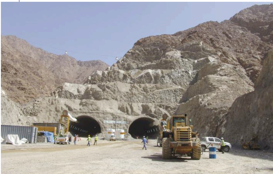
Left: The twin tunnels are the highest in the UAE at 575m above sea level
