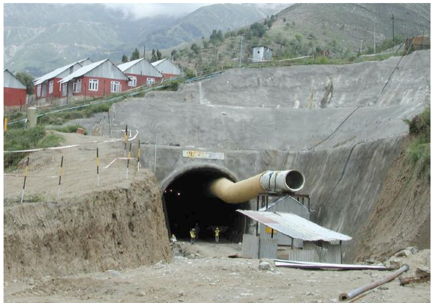
Above: The south portal was excavated in alluvial deposits and slope debris
