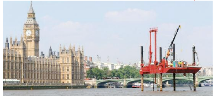
Above: A piling rig works its way up the Thames River to a more accurate understanding of ground conditions for the Tideway Tunnel
