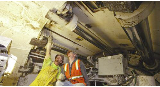
Above left: Two-component back-filling (square window in the tail shield at the top of the photo) reduces risk of subsidence; Below left: Twenty manholes are used for EPB inspection during tunneling
