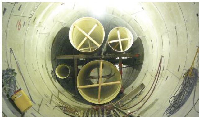
Above: The East contract of the Brightwater conveyance tunnel in King County, Washington, where pipes for several utilities have been placed within the tunnel to maximize usage of free space
