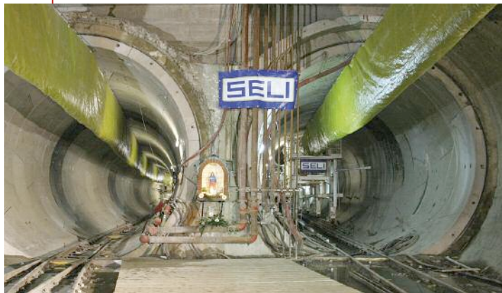
Above: Steady steps taken by Seli on twin TBM drives for Line B1 of Rome metro, and conveyor installation is planned for next month
