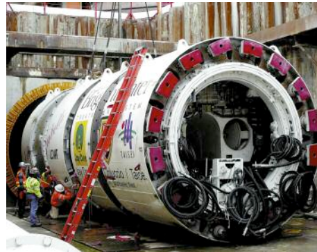
Left: The portal structure at Point Wells and assembly of the BT4 Lovat EPBM prior to launch under the railway
