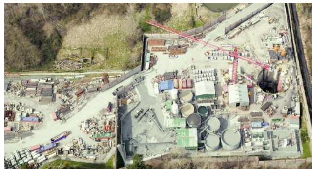
Left: VPFK's North Kenmore site set-up and, far left, launch of the first Herrenknecht slurry machine on the BT2 drive
