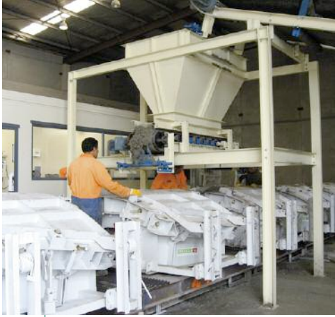
Above: Station for pouring concrete into Ceresola TLS moulds for the Hobson Bay sewer tunnel project
