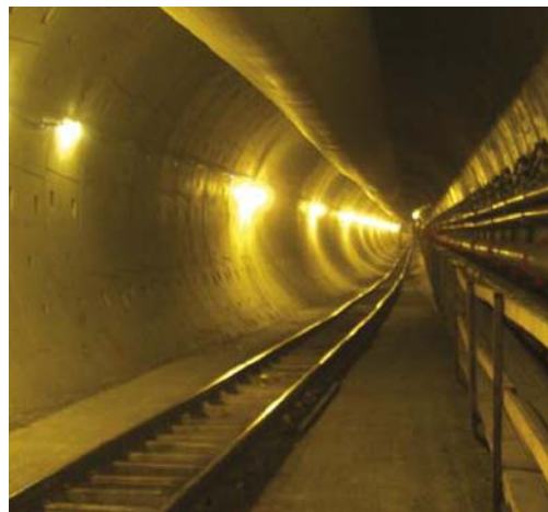
Far left: Figure 1 - Route of the East CSO tunnel and shafts; Top left: The 25ft diameter Herrenknecht Mixshield is readied for launch from Steel Bridge Shaft; Left: View of the universal precast tunnel lining
