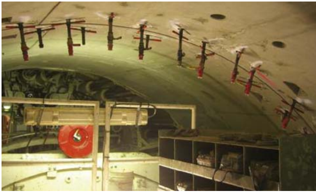
Left: Grout ports mark the tunnel's interface with Steel Bridge Shaft's slurry wall, which was sealed before draining the shaft for free air cutterhead access
