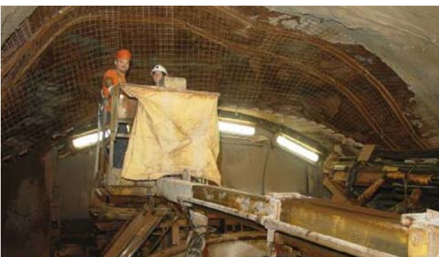
Top left: Fig 1 - Geology along the alignment; Top right: Rowa's L2 ground support area with Meyco robojets; Above right: The crown monorail; Left: One of two boom mounted man-baskets in the L1 area
