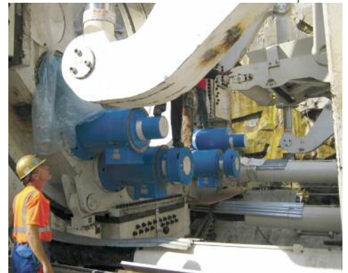
Above: Dave Sethman, Robbins TBM assembly supervisor, oversees the onsite assembly of the 10m diameter Double Shield TBM at AMR
