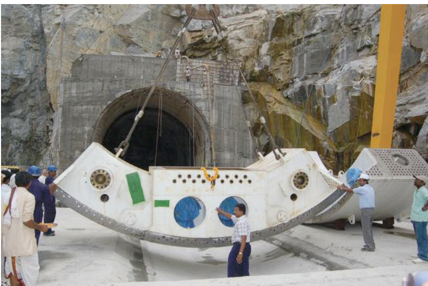
Below: Onsite assembly was used for a Double Shield Machine for India's AMR Project, in Andhra Pradesh state, this May
