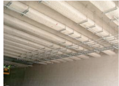
Above: Holmesdale fire protection
