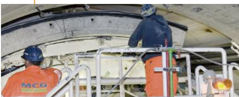
Below: The 7.9m i.d. lining was built with seven segments and a key
