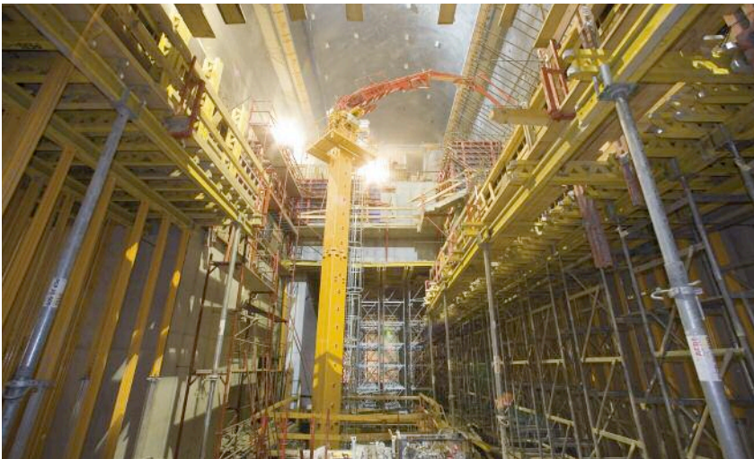
Above: Mammoth concrete pours underway at Kops II, utilising Peri formwork units
