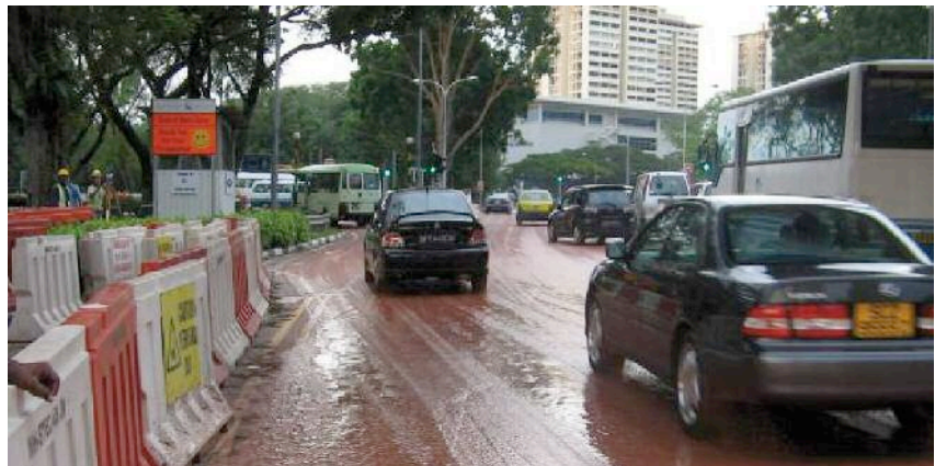
Above: Slurry escape to the surface Right: Fig 3 – The balancing pipes
