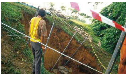
Below: A sinkhole above one of Singapore's deep sewer tunnels
