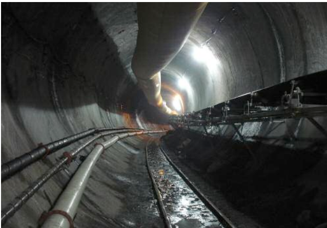
Top: The main conveyor belt, which runs through the East River immersed tube, back to Queens; Middle: Finger hood at the back end of the SELI TBM; Bottom: View along the leading TBM tunnel at up to 120ft (36m) beneath the street's of Manhattan
