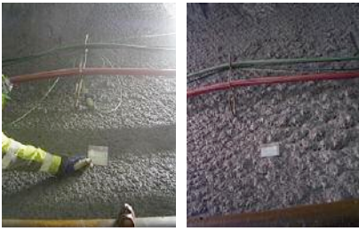
Above: Tunnel wall roughness research in the dominant, TBM-bored parts of Kárahnjúkar headrace was done by establishing surface categories through visual inspections, and some laser scan measurements were undertaken
