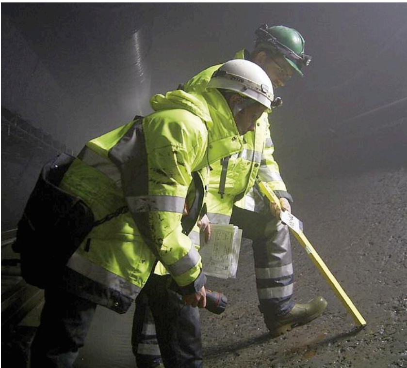
Above: Visual inspection of tunnel wall roughness in Kárahnjúkar headrace during construction to investigate frictional headlosses
