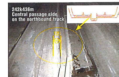
Photo 1 Opening between sub-grade concrete and central passage1)
