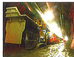
Photo 2 Continuous belt conveyor in the tunnel
