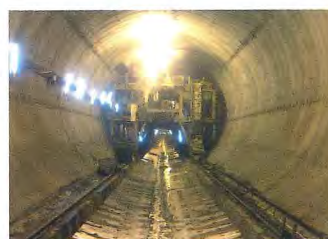
RC liner section of the main tunnel TBM (before placement of the secondary lining)
