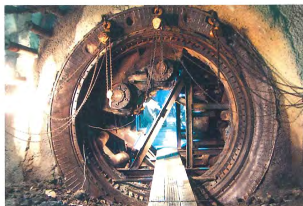
TBM for the evacuation drift broke before reaching the goal
