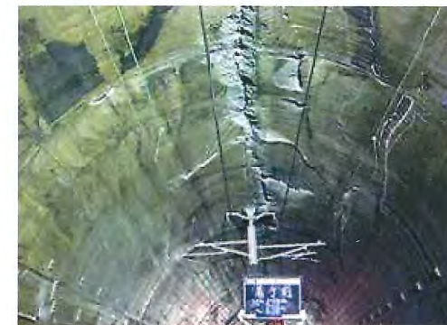
Photo 1 Damage to the Daiichi Yoneyama Tunnel on the Shin-etsu Honsen railway
