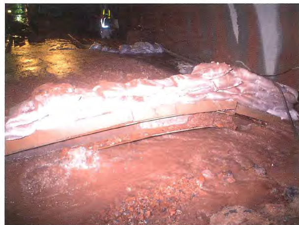
Heaving in the zone without countermeasures
