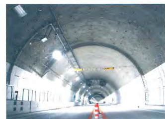
Main tunnel lining with fireproof segments (Front: fireproof segments, Back: ordinary lining)
