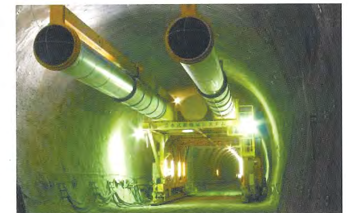
Air curtain ventilation system
