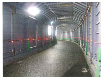
Photo 2 Inside the protector system
