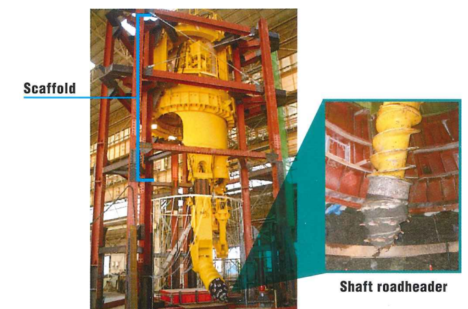
Fig. 2 Photo of the excavation apparatus (roadheader and scaffold) used for sinking a shaft.
