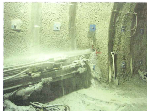
Photo 3 Methane gas blasting out
