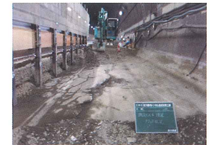
Photo 2 Damage of the old invert
