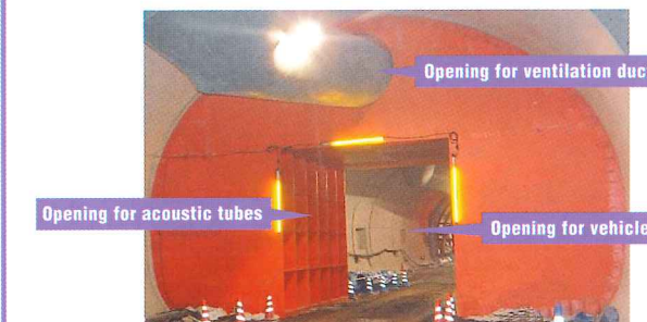
Fig. 1 Blast Silencer ® installed
