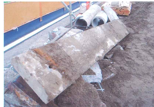
Photo 2 Debris remaining in the reclaimed ground
