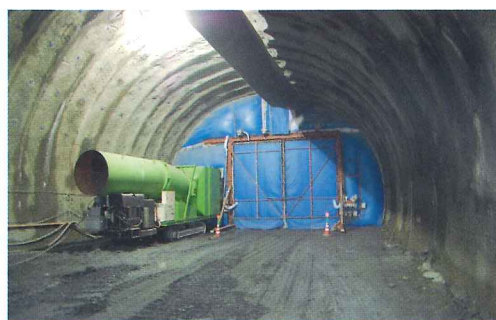
Fig. 2 Electrostatic precipitator and movable balloon bulkhead (view from the portal side)
