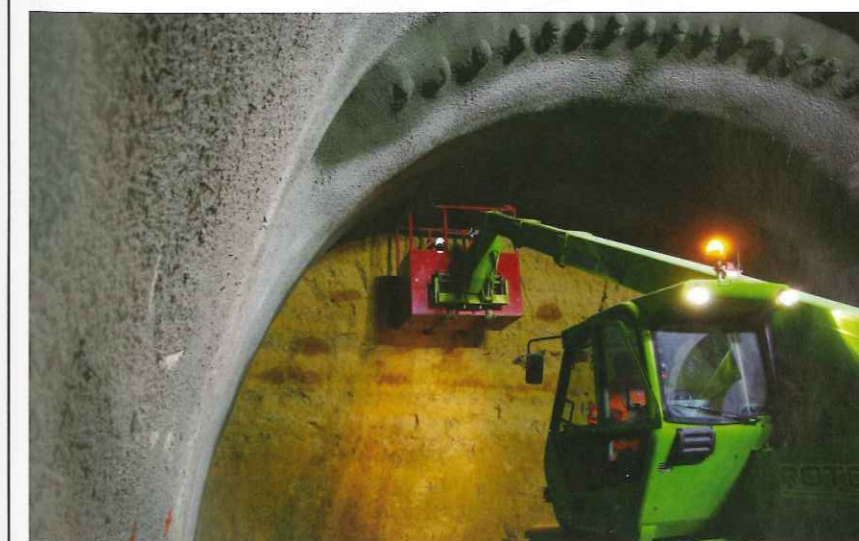
Below: Getting up close to the Hindhead Tunnel face. This allowed detailed face logging and RMR assessment when required
