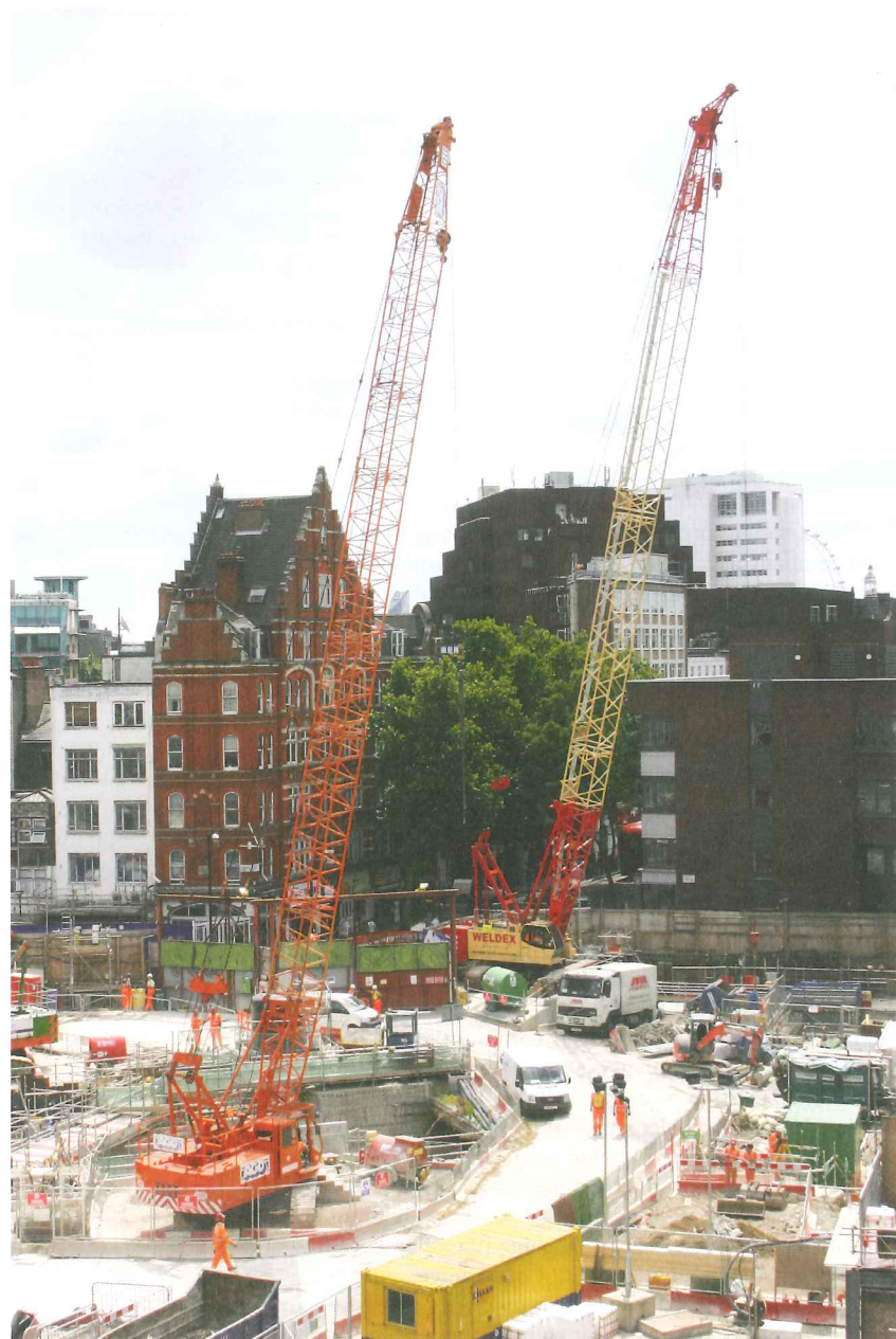
Above: The self weight of wire rope can be a significant factor in lifting work in underground construction
