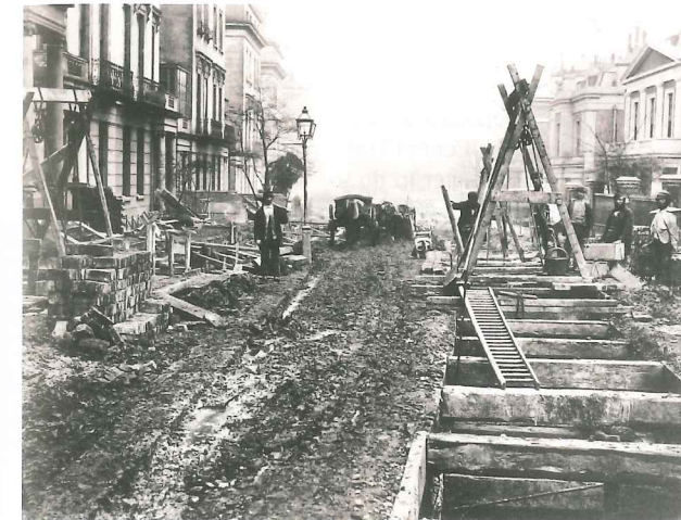
Far left: The line passes from cutting into tunnel. Retaining walls are nearly finished, tunnel arching is already TFL
