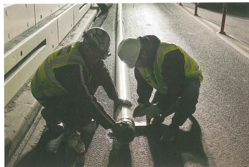
Above (top): Some 1,700 ft (520 m) of pipe and hosing was needed to reach the flood water in the Brooklyn Battery tunnel tubes.
