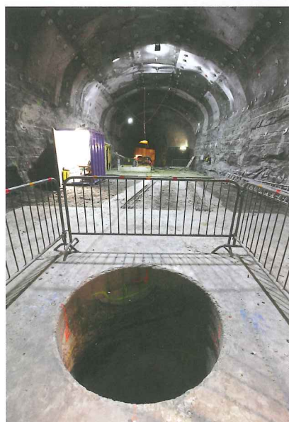
Above: The various sites competed on rock quality and volume of excavation required to create the complex
