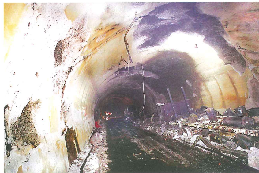
Below: Damaged lining in the Channel Tunnel following the 1996 fire
