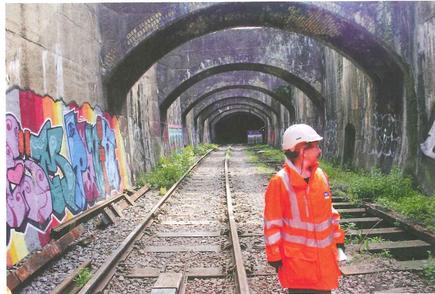
Work is ongoing to refurbish the Connaught tunnel for inclusion in the Crossrail scheme
