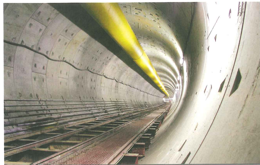
Above: Once complete in 2016, Phase III of the New Delhi Metro extension is projected to carry three million riders annually
