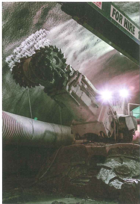
Left: One of the 17 roadheaders used on the Airport Link tunnel project
