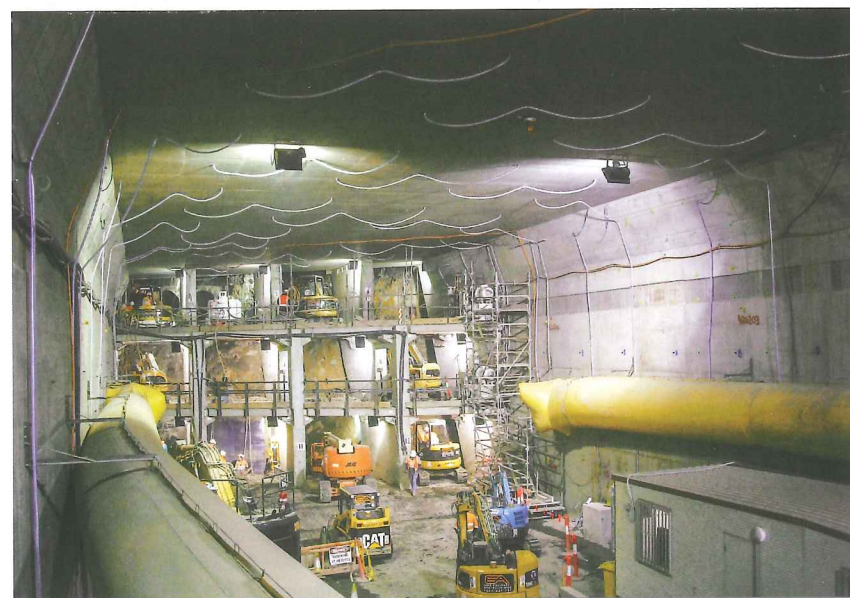
Above (top): The box jack site aerial view showing existing railway infrastructure
