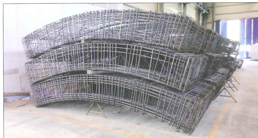
Above: Steel cage bars for the segments had to be reduced in diameter to increase reinforcement
