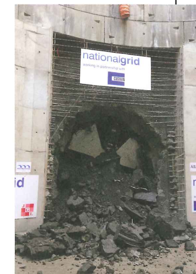
Above: The power tunnels interim breakthrough at Kensal Green before driving on to the substation in St John's Wood
