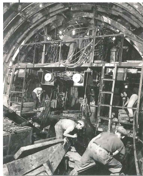
Left: Pick and shovel tunnelling being used for the diversion of the Northern City line at Highbury; the men work within a 16ft (4.9m) diameter hand shield. 20 August 1964. LONDON TRANSPORT MUSEUM
