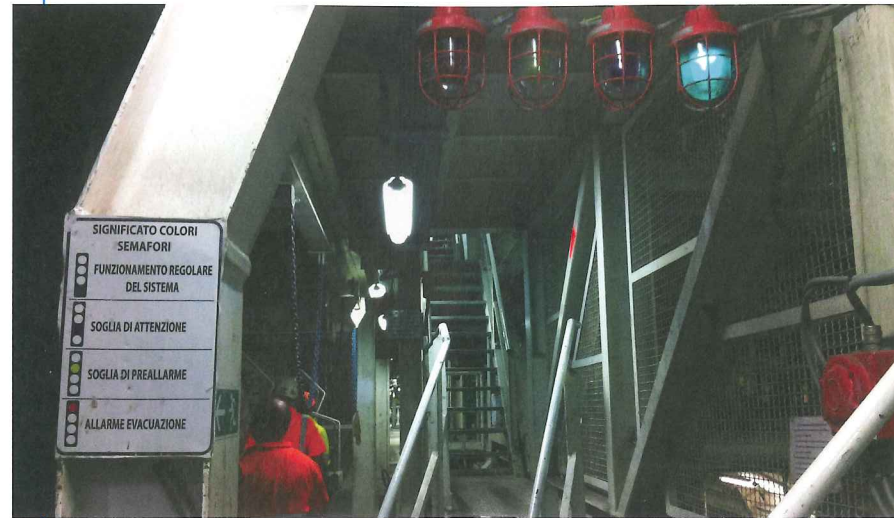
Above: Methane warning system at the lowest alert level, for normal running
