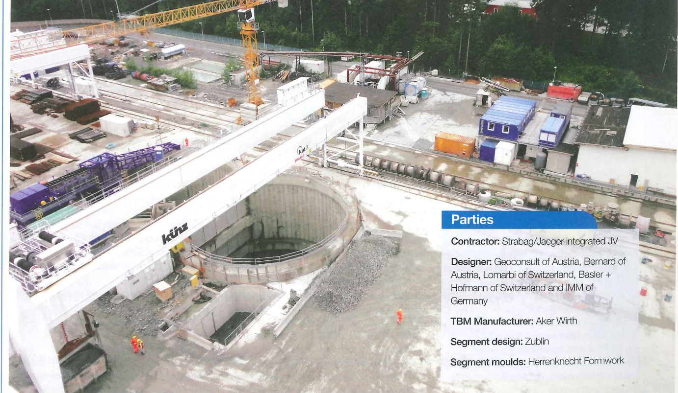
The dual shaft of two 20m diameter cells is 60m deep and constructed with 1.2m diameter secant piles. A gantry crane above is used for muck removal
