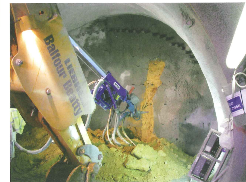
Below: The spray arm advances ahead of the excavator to apply the SCL
