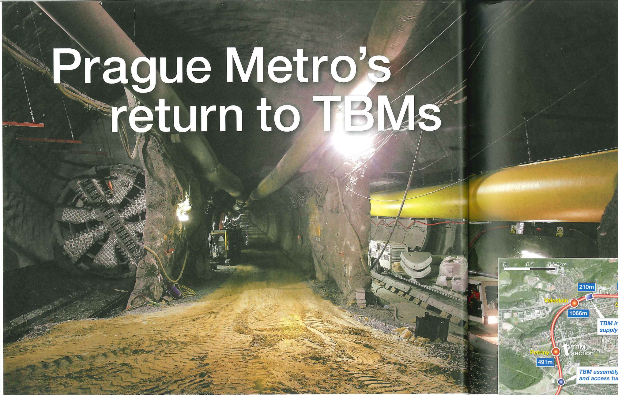
Left: Adela arriving to the one-vault Petřiny Station. Photos courtesy of contractor Metrostav
