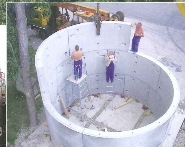
Above: Test ring assembly carried out during segment production at the precast factory
